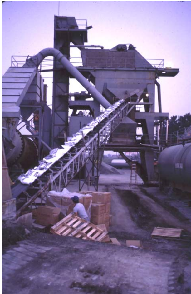
Figure 9 Fibers in Bags on Conveyor to Weigh Hopper
