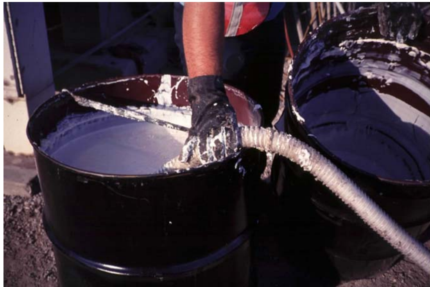
Figure 11 Pumping SBR Latex from Barrel into Plant
